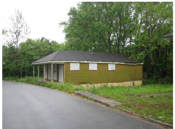
Houses currently occupying the site are in a state of distress and abandonment.
