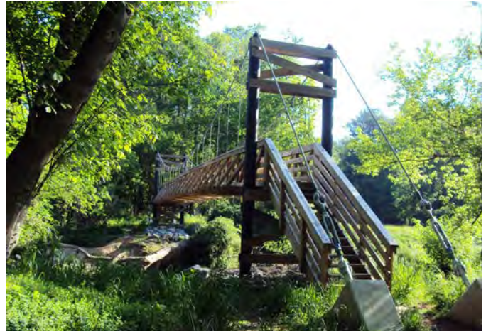
The bridge in Morningside Nature Preserve was designed to withstand flooding. (Segment B)
