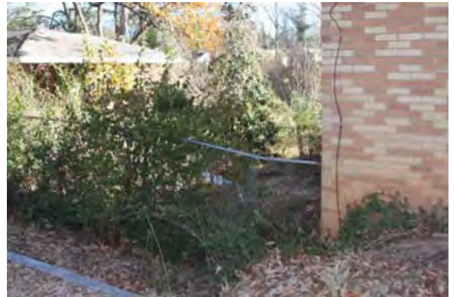
Existing drainage patterns are perilously close to residential structures
